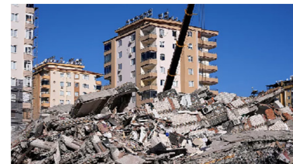
A destroyed residential building in Gaziantep, southeastern Turkey, Thursday, Feb. 9, 2023. © AP Photo
